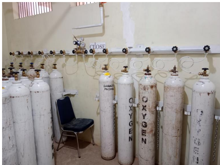
Gambar 7 Instalasi Gas Medik
